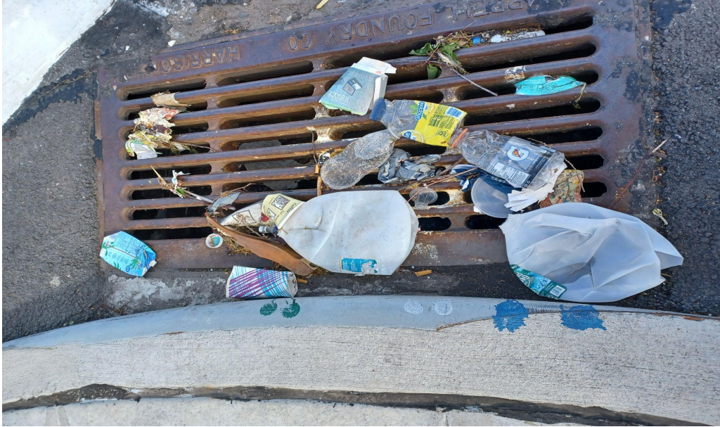
Garbage filled drainage. Barrameda Tsangarides, A. (2023). [Photograph].
